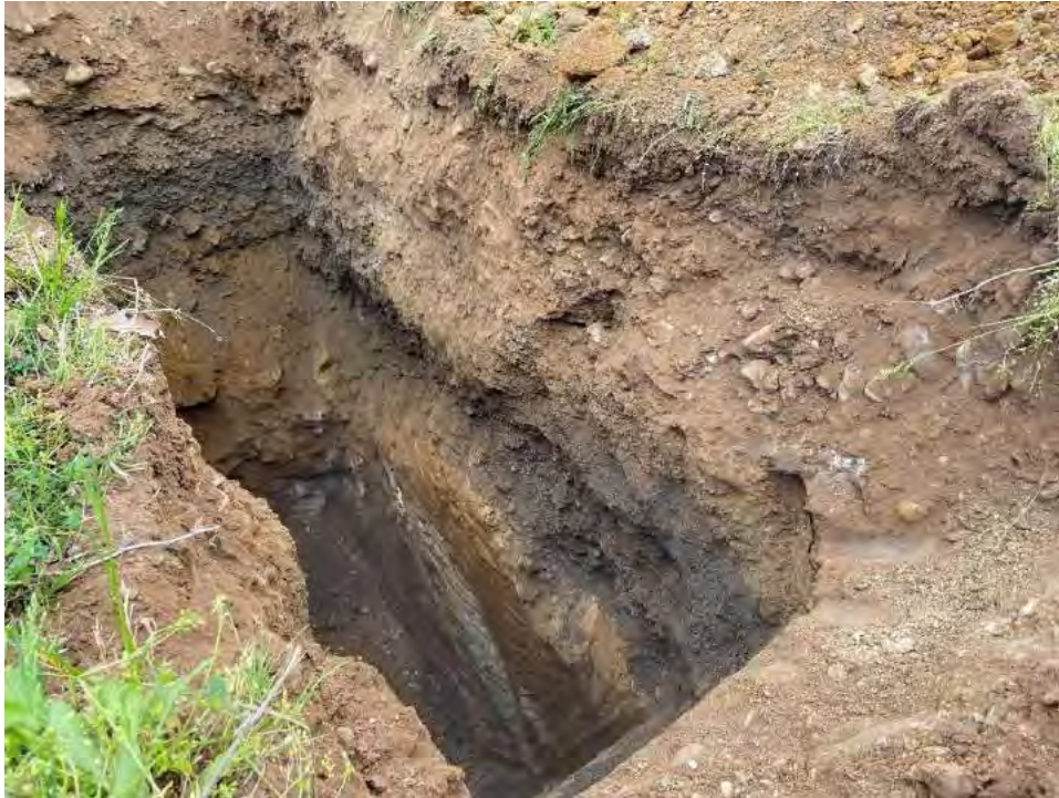
Photograph 5 Test pit with non-indigenous fill material
